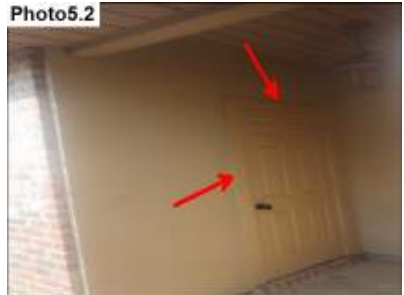
The Side garage door lacks head flashing and sealant joints.
