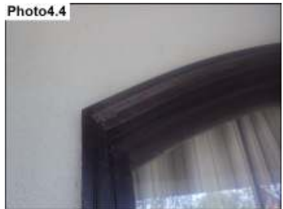
The front door lacks head flashing and sealant joints.
