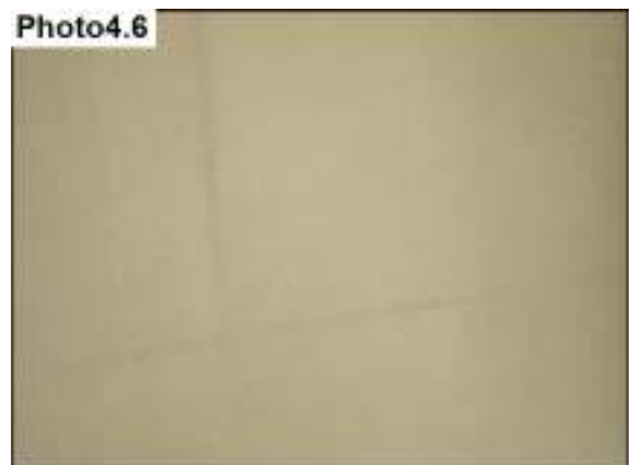
Lines are noted in the stucco wall due to a thin layer of base coat. These lines are the foam boards.
