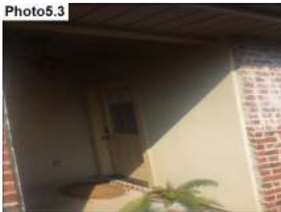
The Side house entrance door lacks head flashing and sealant joints.
