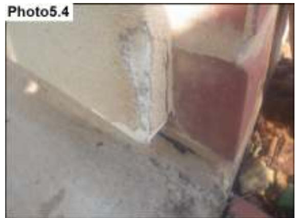
Minor impact damage at the lower right front wall bottom corner.
