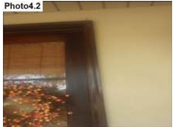
The front window lacks head flashing and sealant joints.
