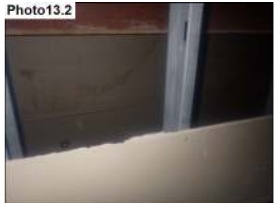
Water stains and damage noted at the back (East) right side upper wall in attic from window leak.
