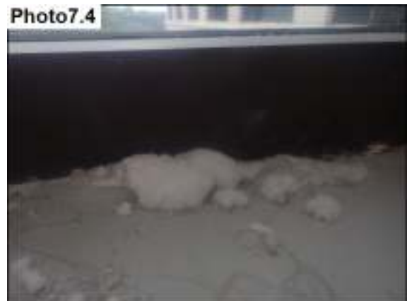
Salt deposits (water damage) from the elevated moisture in the plaster of the front entrance windows.
