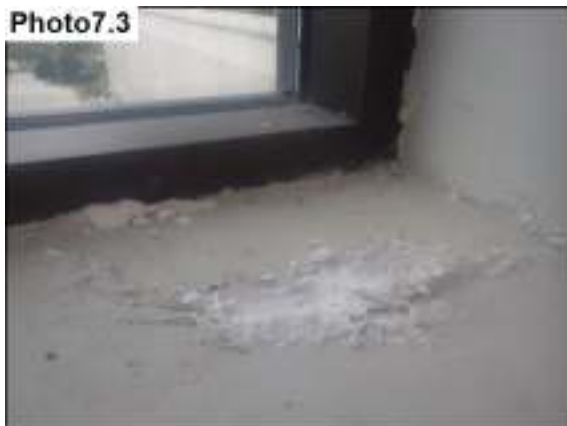
Salt deposits (water damage) from the elevated moisture in the plaster of the front entrance windows.
