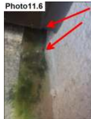
Leaking at the bottom of the Back Entrance East facing window. Sealant Joint photo.
