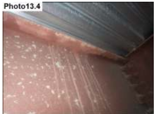
Water stains noted at the front (West) left side upper wall in plenum space from window leaks.
