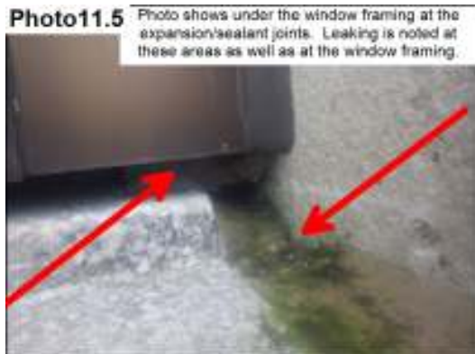
Leaking at the bottom of the Back Entrance East facing window. Sealant Joint photo.
