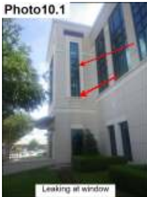
Back Entrance right side upper window leaks at the base
