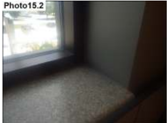
Office Space 209J interior view. No water damage at the sill or drywall noted at this time.
