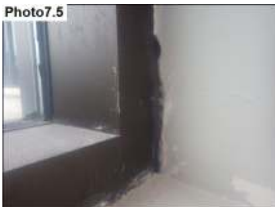
Large crack at the bottom of the front entrance windows; repair after the leaking is corrected.
