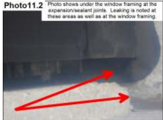
Leaking at the bottom of the Back Entrance East facing window. Bottom of window photo.
