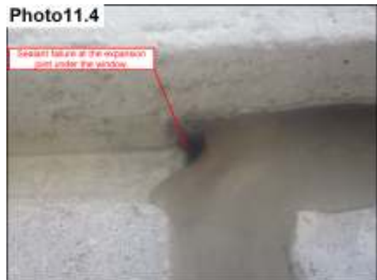
Leaking at the bottom of the Back Entrance East facing window. Sealant Joint photo.
