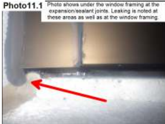
Leaking at the bottom of the Back Entrance East facing window Bottom of window photo
