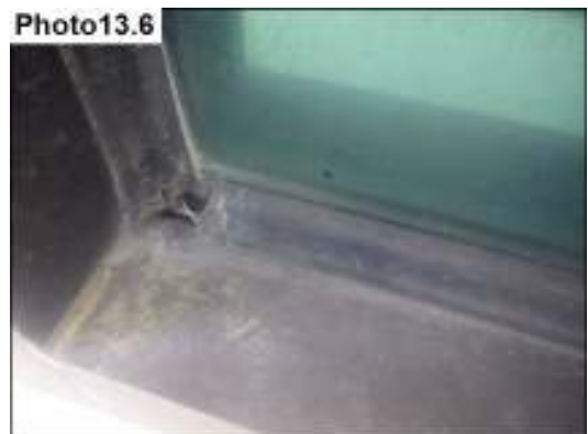
Gasket failure at the exterior side of the windows.
