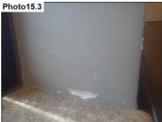
Small area of water damage at the side wall of the second floor office space 212F (Alex Calomb).
