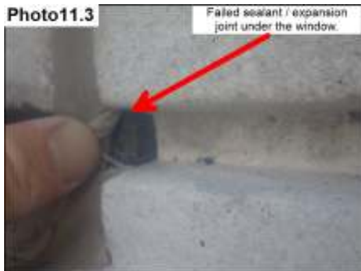
Leaking at the bottom of the Back Entrance East facing window. Sealant Joint photo.
