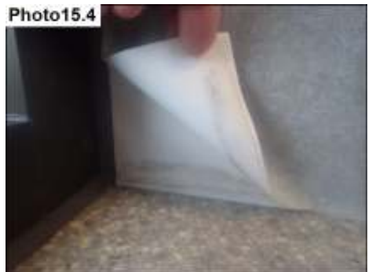
Upstairs break room water damaged wall with apparent microbial growth; correct and repair
