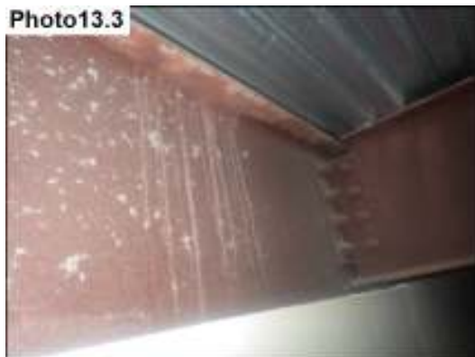
Water stains noted at the front (West) left side upper wall in plenum space from window leaks.
