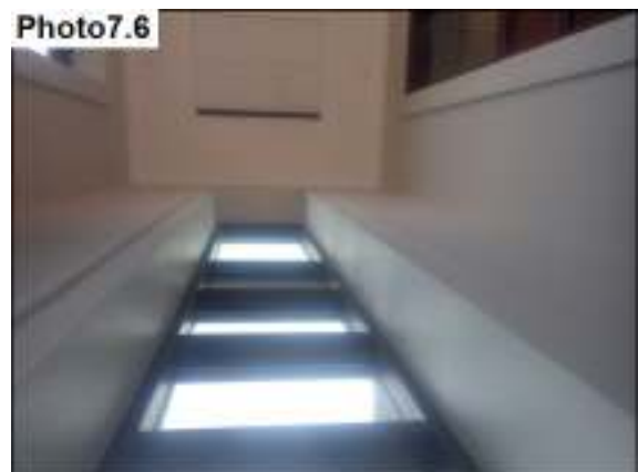
The vent at the ceiling is cooling the window frame, which allows condensation at the window.
