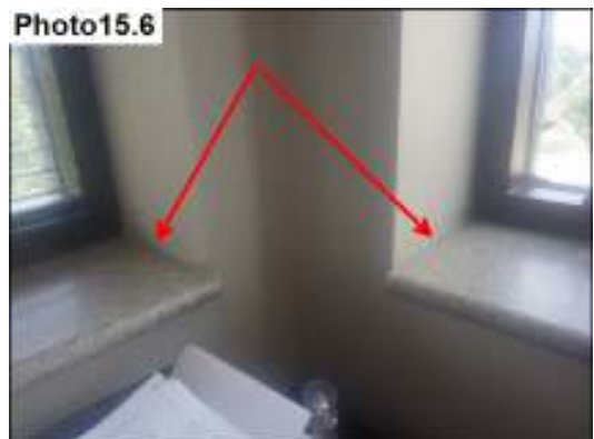
Water stains and damage is noted at the second floor window likely due to condensation.
