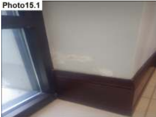
Minor water damage at the lower Back entrance windows
