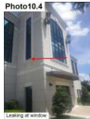
Back Entrance left side upper window leaks at the base.
