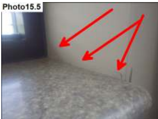
Water stains and damage is noted at the second floor window likely due to condensation.
