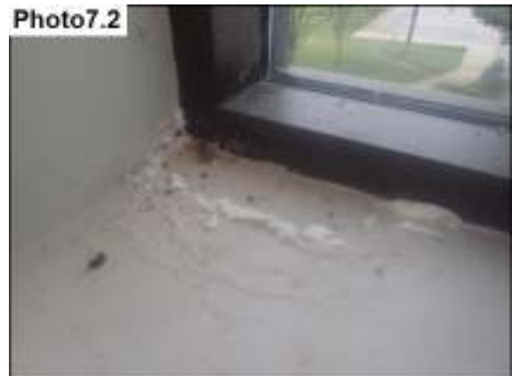
Salt deposits (water damage) from the elevated moisture in the plaster of the front entrance windows.
