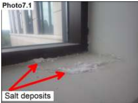
Salt deposits (water damage) from the elevated moisture in the plaster of the front entrance windows
