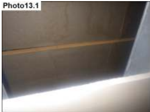
Water stains and damage noted at the back (East) right side upper wall in attic from window leak
