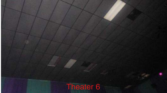
Photo #7: Water damage and entry inside Theatre
